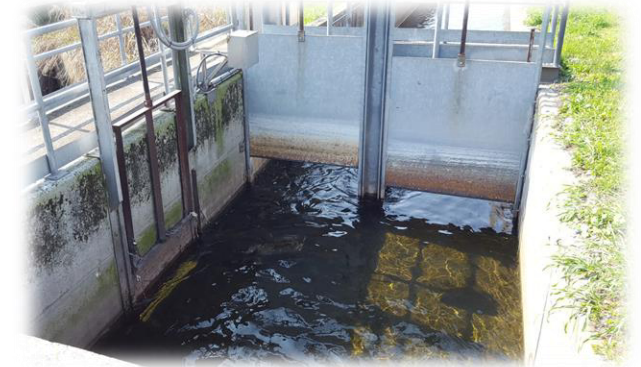
Gate openings and VF levels
